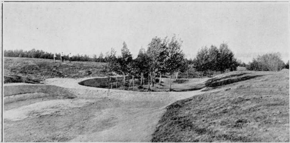
Golf in the North Country. The water hazard under construction on No. 2 Fairway of the sporting new course at Haileybury, Ontario.
